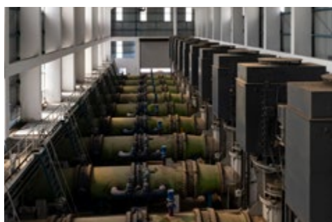
A pumping station constructed as part of the ADB-funded project that will channel water to distribution chambers with onward transmission to farmers' fields.
