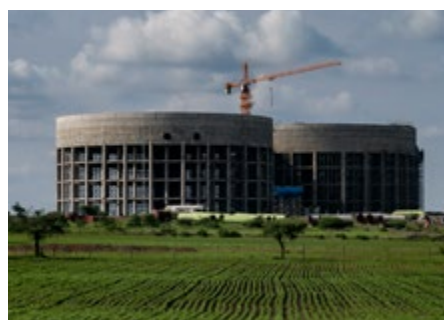
A distribution chamber that will transmit water to farmers' fields by gravity.
